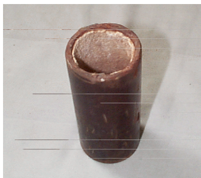
Figure 2. Scale in a cut-out section of tubing showing how it is deposited inside the unprotected pipe.
